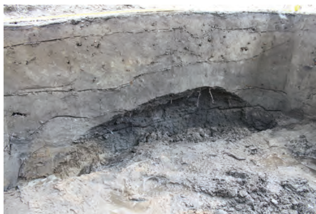
Figure 4-13. Portion of the south wall of N183E12 that collapsed minutes after being re-excavated and troweled for photography.
