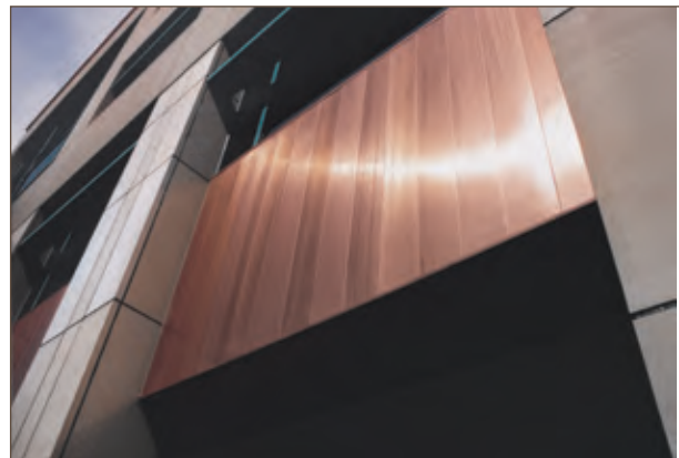
Figure 3.3A. The Anchor Center office building in Scottsdale, Arizona, chose to boast its location in the Copper State by preserving the natural color of freshly milled copper sheet with a clear coating. Due to sun and heat, the finish requires reapplication every few years to maintain its pristine look.
